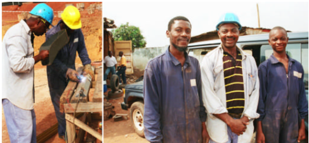
The owner of Boyo Atelier, a welding shop, has been building up his business based on an on-call arrangement with the contractor preparing the site for Pump Station 3 near Bélabo. Pascal Endong Bolomiqui is shown here supervising one of his workers at the job site, and in front of a new vehicle he has bought so he can take his new welding unit to job sites. He reports that he had to improve his welding technique in order to get the work and as a result of working with the Project's contractors he has learned how to follow drawings when fabricating items.
