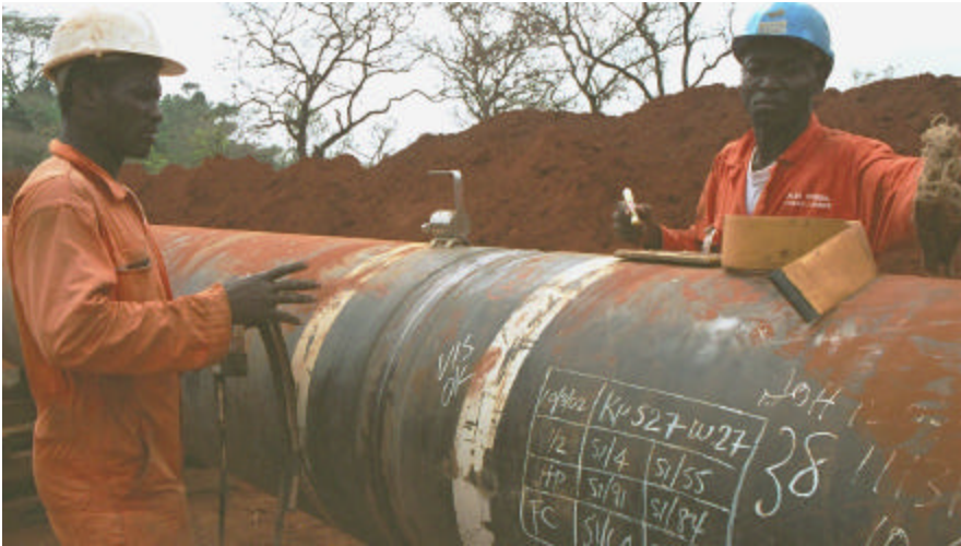
Technicians from the Cameroonian company Hydrac perform a radiographic test on a weld in the pipeline under construction in northern Cameroon. Hydrac, a Douala-based laboratory and non-destructive testing firm, has contracts for this and other types of testing with several of the Project's contractors.
