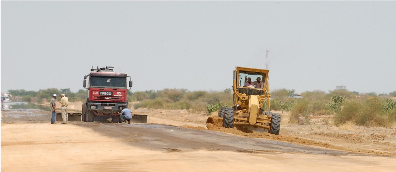
The old dirt track road to Abeché will be paved by this road construction project. The all weather road will have a solid base built of laterite augmented by cement. It is being paved with asphalt. Project revenues will fund the construction, the first project to be made possible by the oil revenues.
